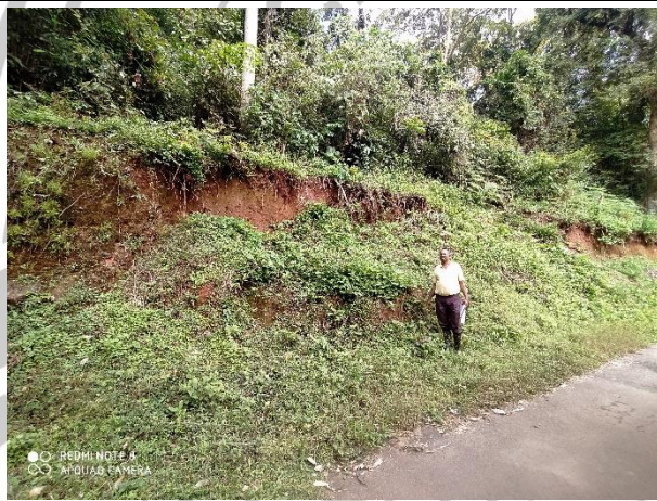
I) Cut slope failures along Kirudale road section ( 12^{\circ} 32' 42.31''\text{N}/75^{\circ} 48' 5.93''\text{E} )
