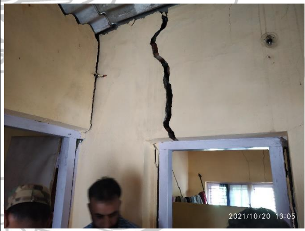
L) Development of cracks on the wall at Biligeri Ghandi house ( 12^{\circ} 27' 28.33''\text{N}/75^{\circ} 48' 26.83''\text{E} )
