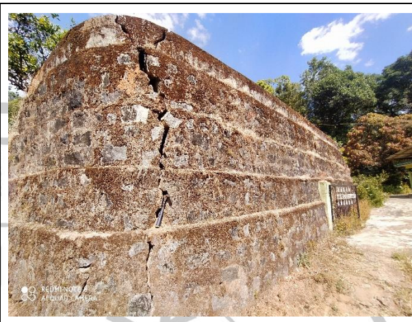
H) Developments of the cracks on the drying yard in and around Garwale ( 12^{\circ} 33' 38.96''\text{N}/75^{\circ} 47' 3.95''\text{E} )
