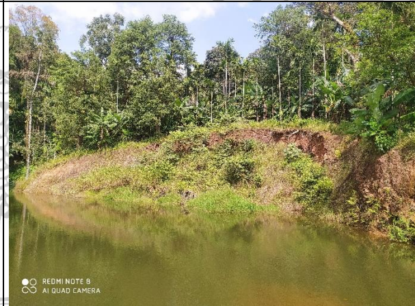
D)Cut slope failure ( 12^{\circ}33' 1.51''\text{N}/75^{\circ}47' 42.73'' \text{ E} )
